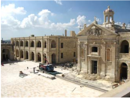
Figure 6. Recent view of the restored St Anthony's Chapel and the adjacent Barrack Blocks.
